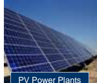
PV Power Plants (> 100 kW)
